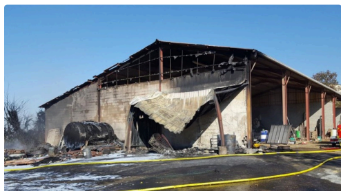
pompier gaz oil 3.JPG
